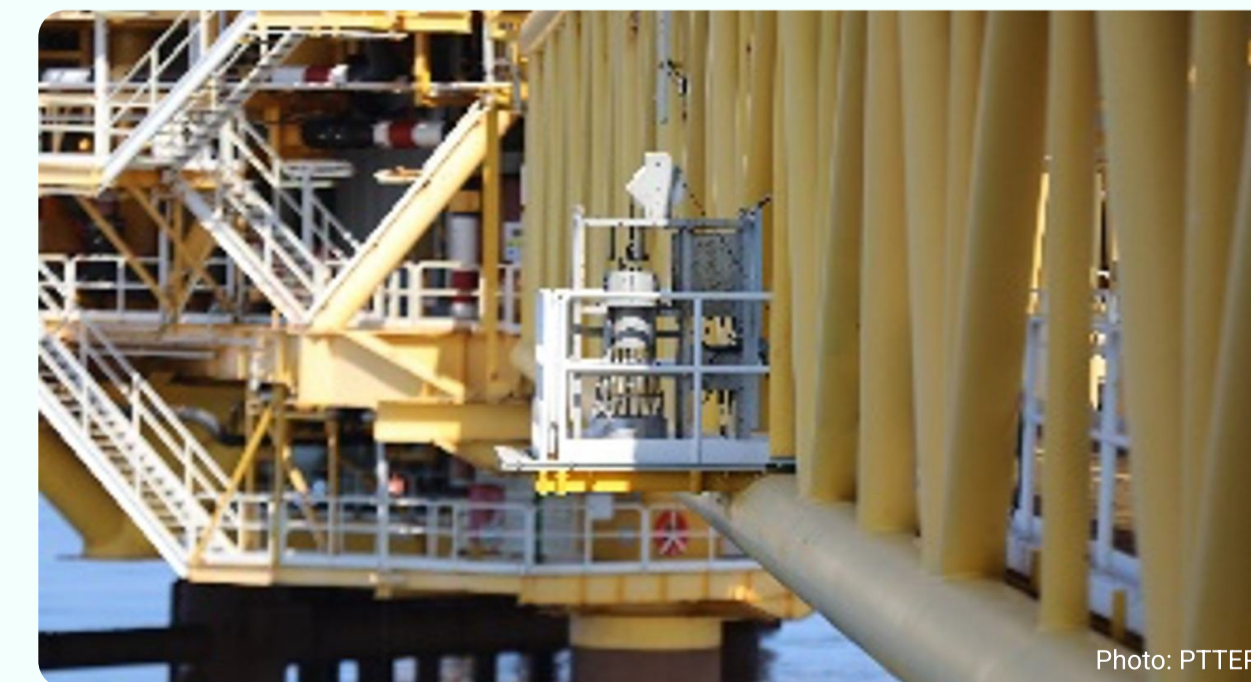
Picture 1. Photo of Telemetry Marine Monitoring System
